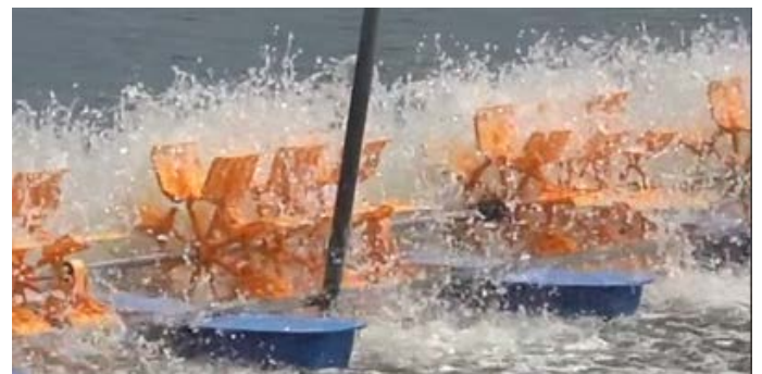
Operation of aeration unit
