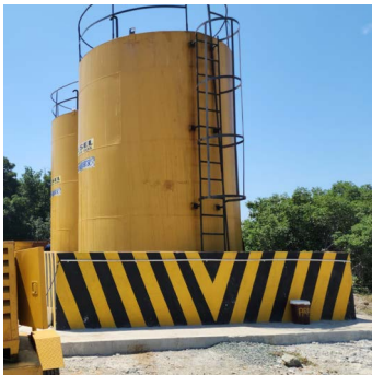
Main fuel tank
